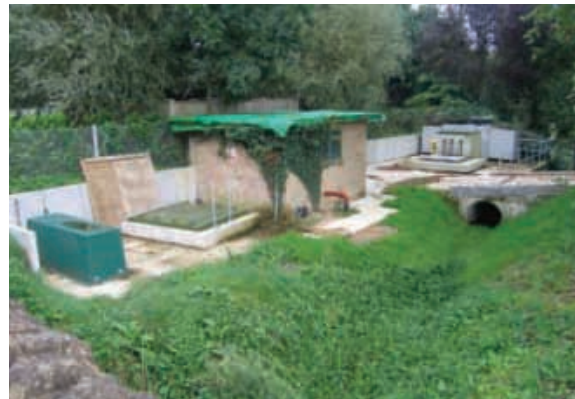
Water pumping station.
