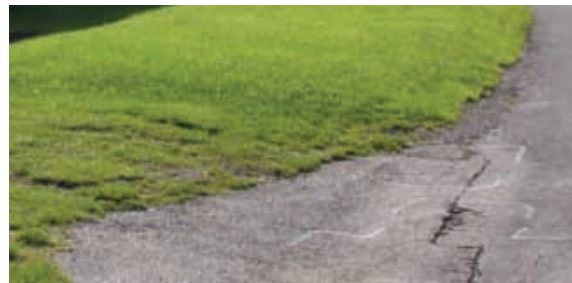
Grassed verge meeting edge of road . Road surfaces shows signs of patched repairs
