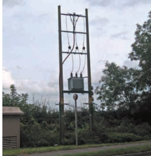
Transformer adjacent to Fir Tree Farm.
