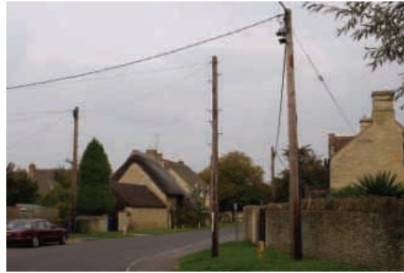
Overhead cables on Church Lane.
