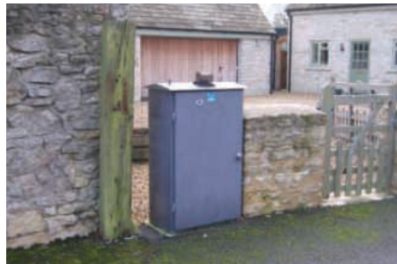
Service equipment placed within boundary wall facing onto footway.
